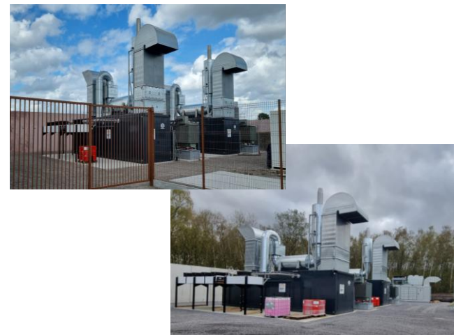
Installation completed for the 4 CHPs (Angres and Rouvignies) in France
