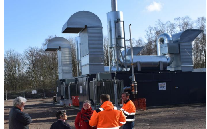
Installation completed for the 2 CHPs in Angres site
