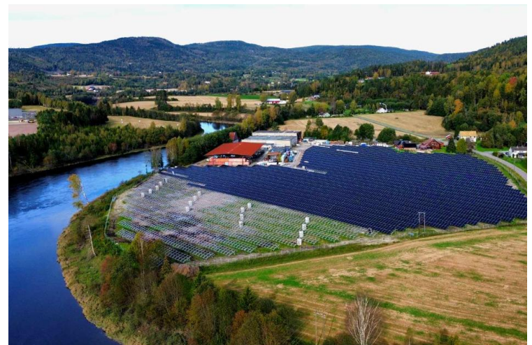
Installed solar photovoltaic panels in Engene, Norway
